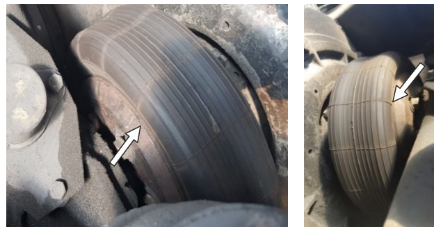
Figure 5. Motor car ER2 991-02 – incorrect installation of the rubber-cord coupling
