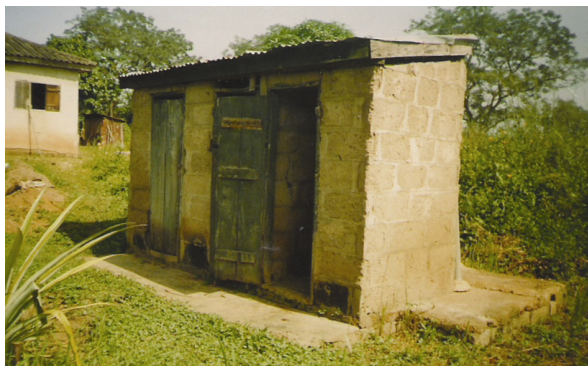
Fig. 5. Front view of the pit latrine in camp 2 where flies tend to breed due to exposure from a damaged door
