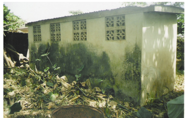
Fig. 3. View of behind the bathroom in camp 2 where wastewater percolates directly into the soil
