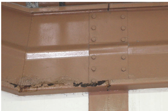
Fig. 1. Corrosion attack on cold-formed beam in an urban atmosphere, sheltered exposure, Naples (Italy)
