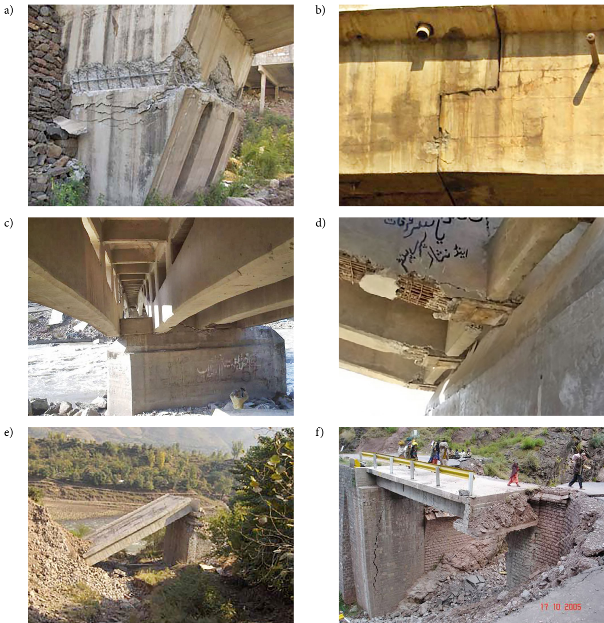
Figure 5. Some damages to bridges during 08 October, 2005 Kashmir earthquake: a – Severely damaged abutment, Garhi Dopata bridge; b – bridge pounding at expansion joint, Garhi Dopata; c – Balakot bridge over River Kunhar, Balakot City; d – Spalling & cracks in Balakot bridge; e – Drop down of Sobri Bridge, Mzd Sri Nagar Road; f – Abutment failure of a bridge in AK
