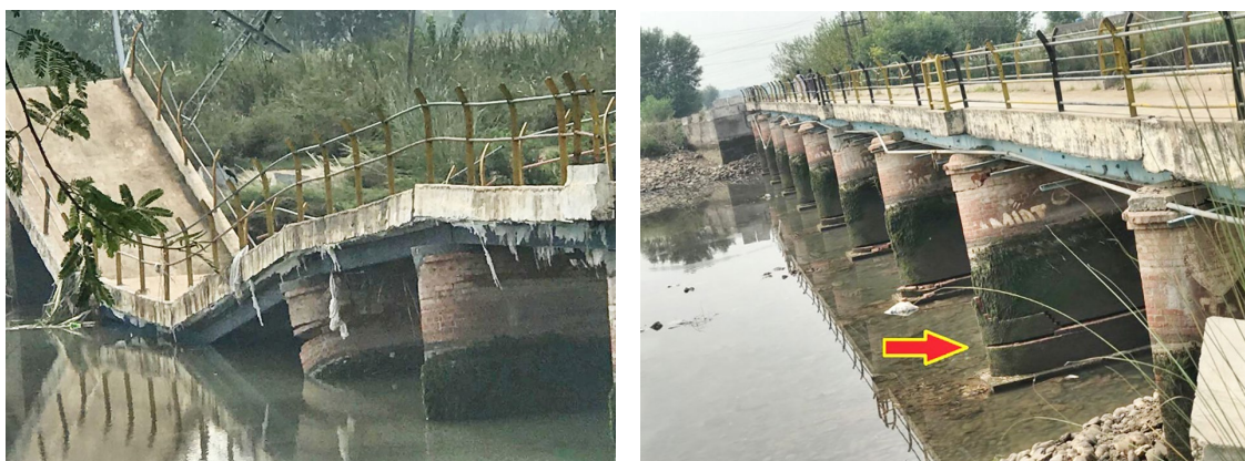
Figure 7. The damages of bridge on Jatlan canal during September 24, 2019 earthquake
