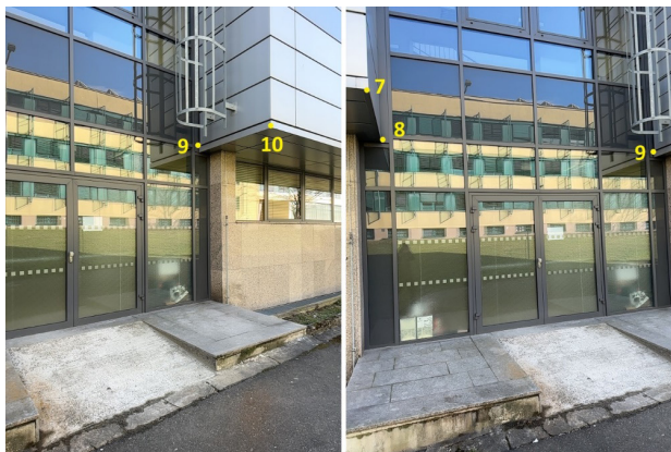
Figure 10. Problematic points on the building
